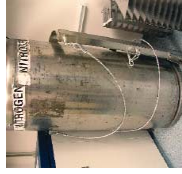
Seismic restraint of Liquid Nitrogen tank
